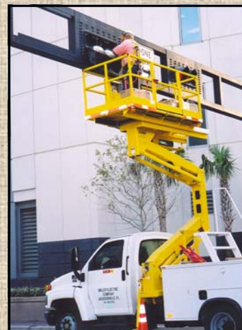
Above: Electrician changing out lamps in a signal head and replacing with LED.
